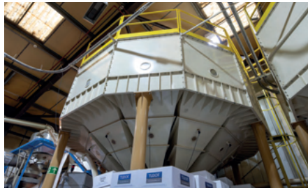
Green Coffee – Raw – Storage Silos
